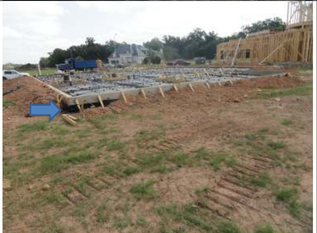
PHOTO 16 COMPACT GRADE MATERIAL AT MASTER BEDROOM FORM BOARD SO CONCRETE DOES NOT DRAIN OUT
