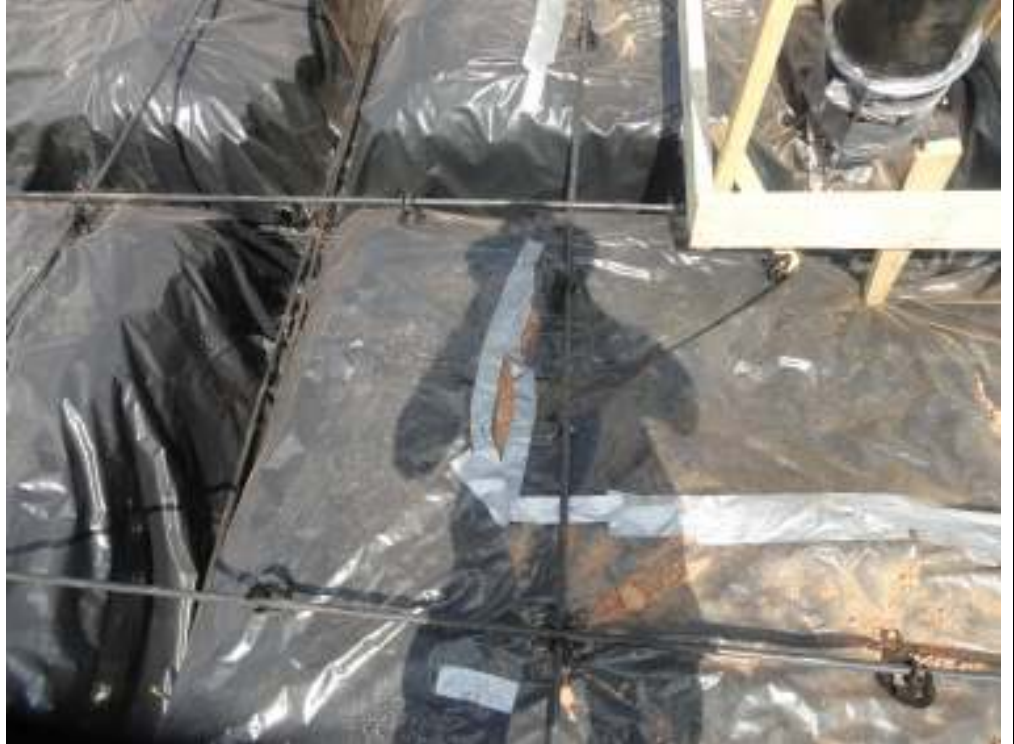
PHOTO 9 POLY TEAR NEEDS TAPE AT MASTER BATH AREA
