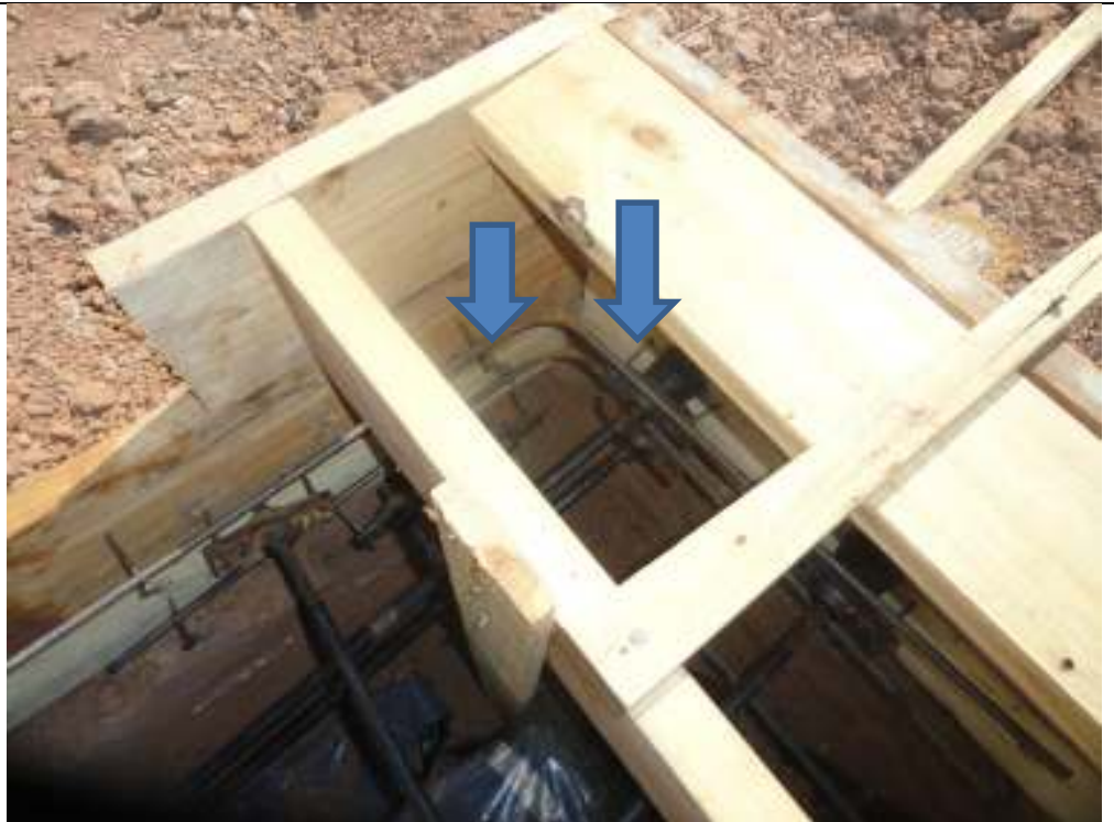
PHOTO 2 ANCHOR NAILERS MUST BE AT LEAST 6" AT EDGE FROM GARAGE CORNER
