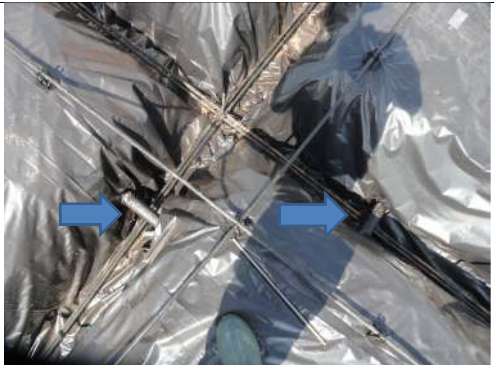
PHOTO 4 TAPE UP POLY WRAP TEARS AROUND PLUMBING BETWEEN KITCHEN AND GARAGE
