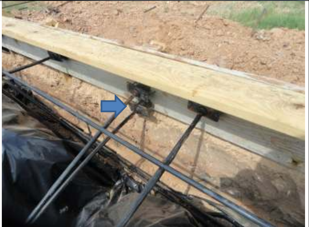
PHOTO 12 POCKET FORMER MUST BE FLUSH AGAINST FORM BOARD AT MASTER BEDROOM SIDE WALL
