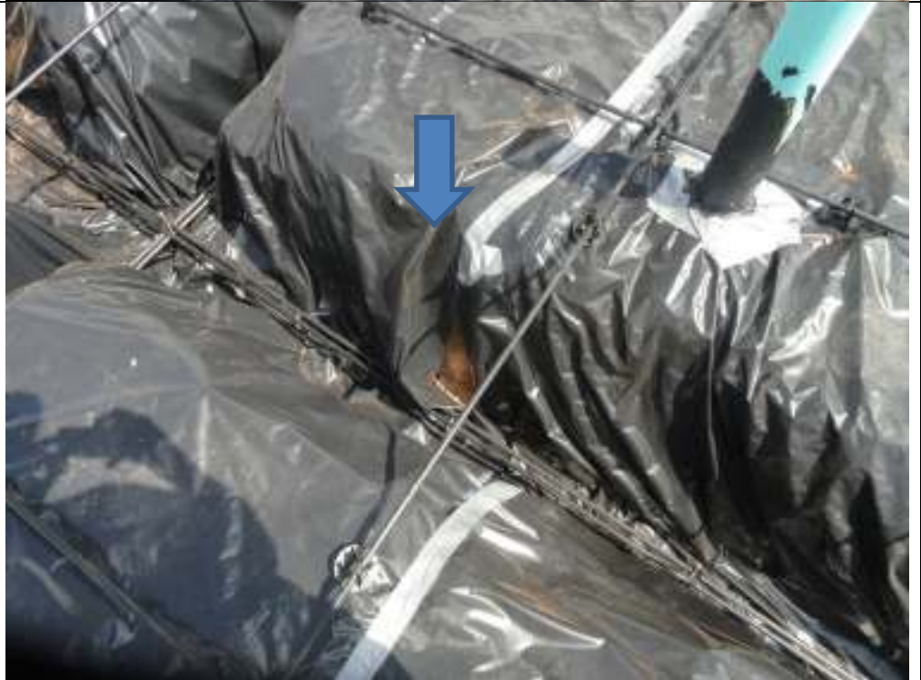
PHOTO 10 OVERLAP 12" AT JOINT AND FULLY TAPE POLY WRAP AT COURTYARD DRAIN BEAM
