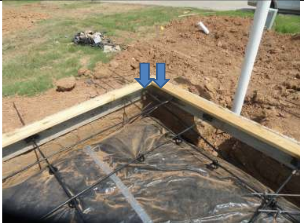
PHOTO 15 ANCHOR NAILERS MUST BE AT LEAST 6" FROM SLAB CORNER AT FRONT LIVING WALL
