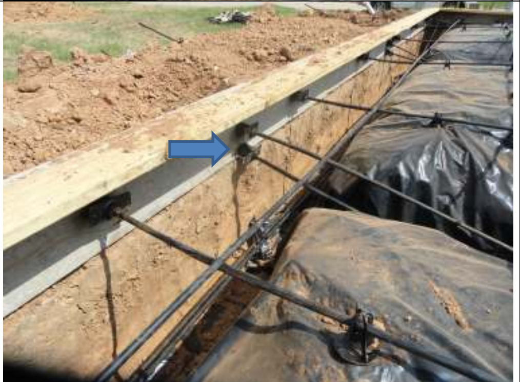
PHOTO 14 POCKET FORMER SHOULD BE FLUSH WITH FORM ON MASTER BATH WALL
