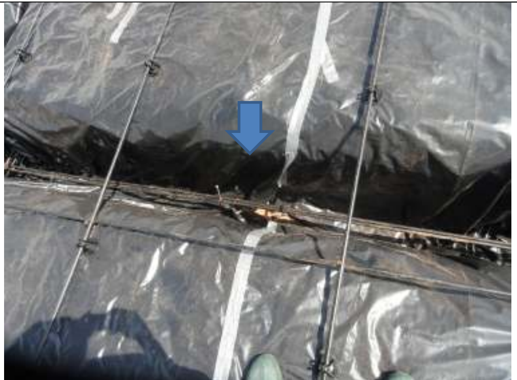
PHOTO 8 NEAR CENTER OF FORM POLY JOINTS MUST BE OVERLAPPED A MINIMUM OF 12" AND FULLY TAPED TO SEPARATE FROM BARE SOIL
