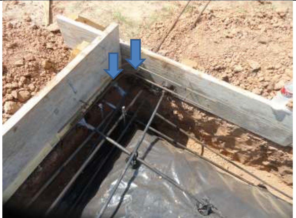
PHOTO 7 REAR PATIO CORNER ANCHORS NEED AT LEAST 6" DISTANCE FROM EDGE FOR STRUCTURAL STRENGTH
