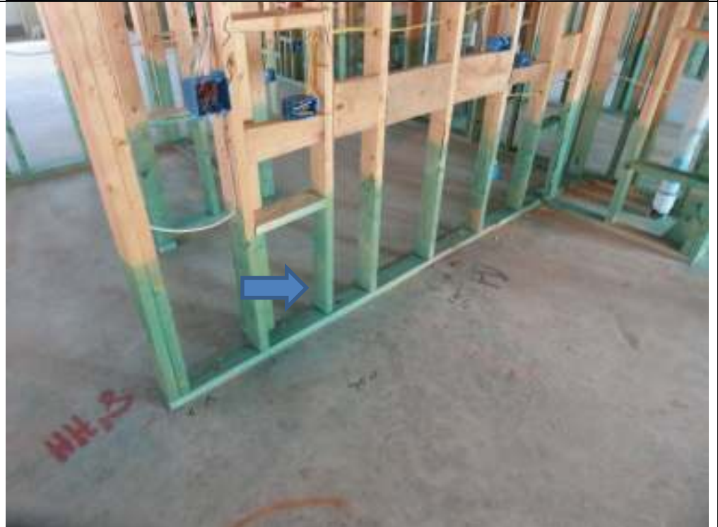
PHOTO 18 RECESS KITCHEN STUD EVEN WITH EDGE OF BOTTOM PLATE SO DRYWALL WILL NOT BE WAVY
