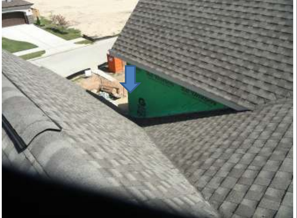
PHOTO 7 RECOMMEND PAN METAL AND STEP FLASHING BE INSTALLED AS ROOF VALLEY TERMINATES INTO WALL
