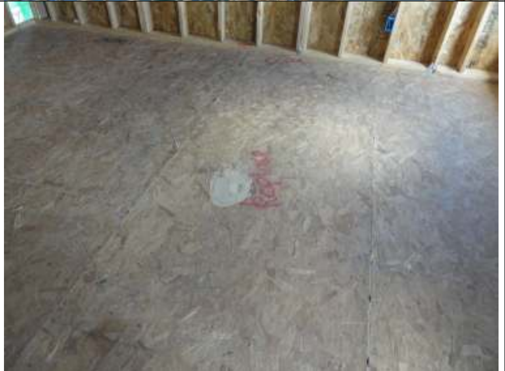
PHOTO 20 UPSTAIRS BEDROOM (OVER MASTER BATH) FLOOR OSB SHOULD HAVE NEW PIECE INSTALLED DUE TO HOLE. FLOAT MATERIAL IS INSUFFICIENT
