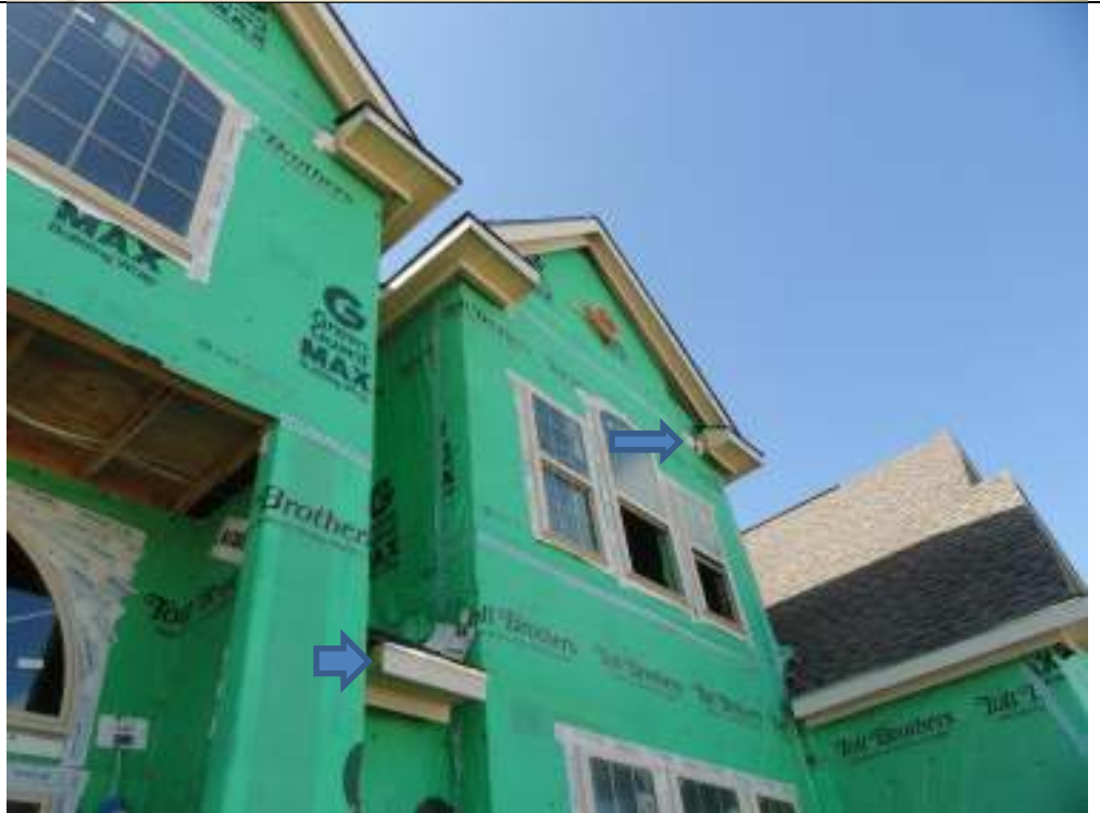
PHOTO 2 FLASHING TAPE NEEDED
