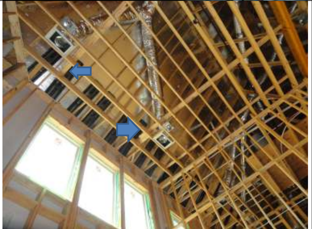
PHOTO 16 FAMILY ROOM RAT RUNS MUST BE NAILED TO RAFTERS TO PREVENT TWISTING OF JOISTS
