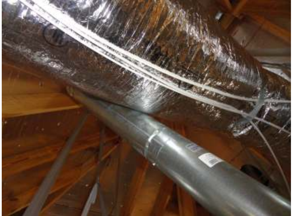
PHOTO 23 1" CLEARANCE NEEDED FROM DUCT FOR FURNACE FLUE PIPE
