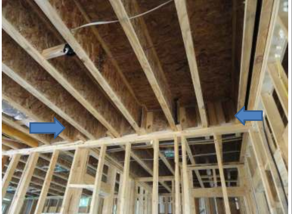
PHOTO 13 GARAGE WALL (ADJOINING PANTRY) NEEDED MORE FOAM SPRAY SEALANT FOR AIR LEAKAGE
