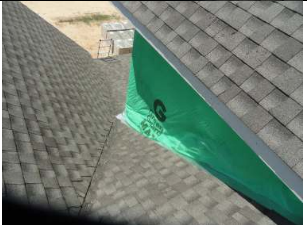
PHOTO 8 SAME AS LAST PHOTO (AREA OVER MASTER BEDROOM AND CLEAN OFF ROOF OF EXCESS NAILS AND OTHER DEBRIS
