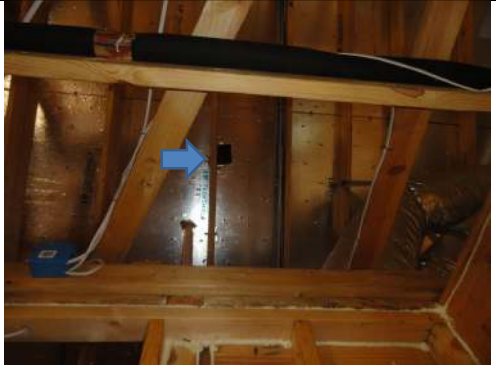
PHOTO 21 DECKING REPAIR TO FILL IN CUT OUT (OVER CLOSET OVER MASTER BEDROOM HALL) NEEDED TO PREVENT STEP THROUGH ROOF
