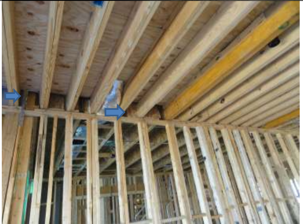
PHOTO 10 FOAM SEAL SPRAY NEEDED AT GARAGE (IN CERTAIN AREAS)
