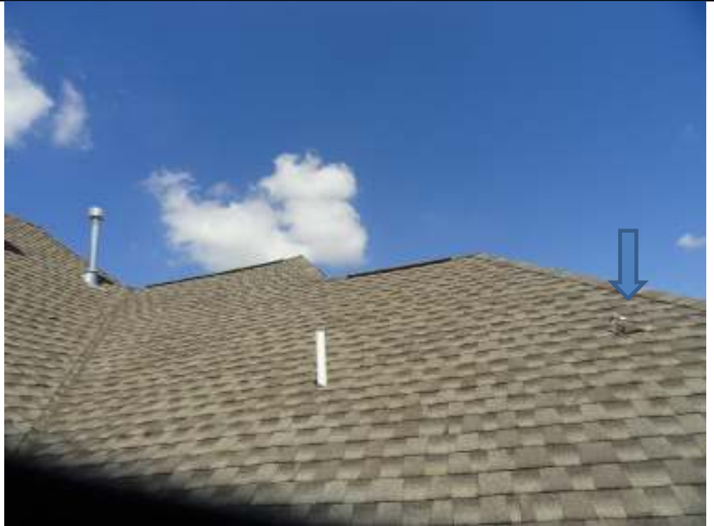
PHOTO 9 UPSTAIRS BATH (OVER MASTER BATH) EXHAUST FAN VENT PIPE MUST TERMINATE THROUGH ROOF
