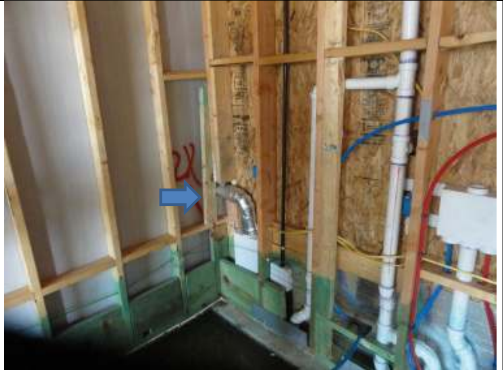
PHOTO 15 GUEST BATH CORNER WALL NEEDS A FULL 2X6. IT SHOULD EXTEND UNCUT FROM FLOOR TO TOP PLATE
