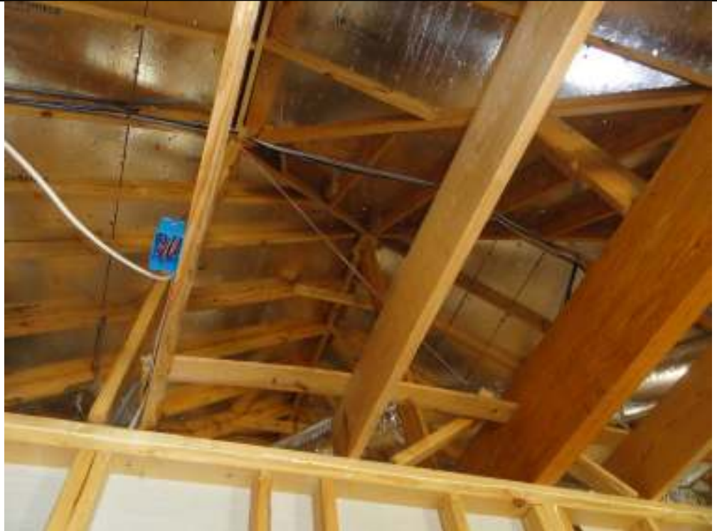
PHOTO 25 DECKING MUST BE CUT BACK AT LEAST 1" ALONG ENTIRE BOTH SIDES OF PEAK RIDGE VENT (OVER STAIRWELLS)
